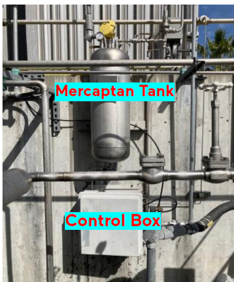
Mercaptan feed control equipment at WM El Cajon Hauling to be replaced.
